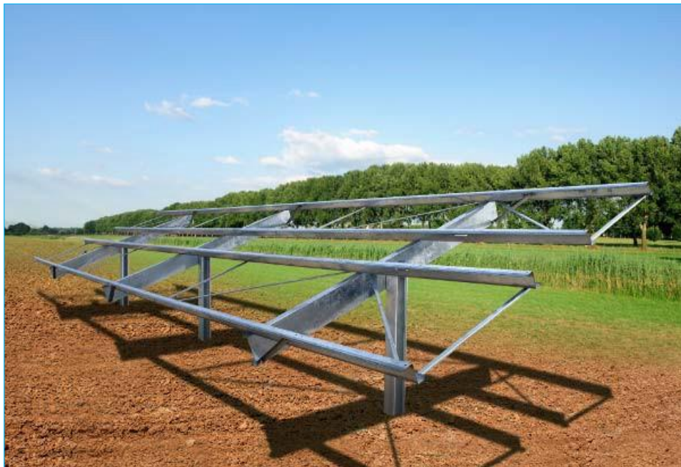
Plate 2.4: Example of a solar PV support structure
